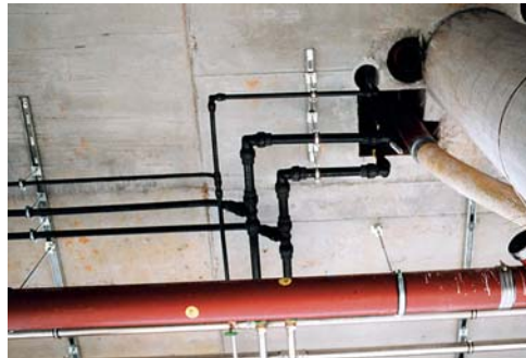
6800 metres MT pipes serving as the mains riser pipe and as the distributing branches.
