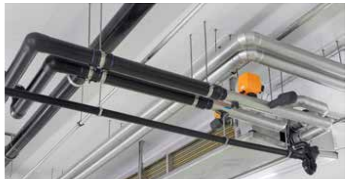
All components of the pipe cooling system are already pre-insulated.
