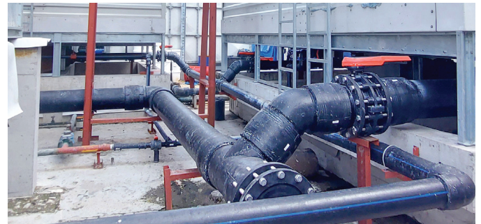
Bare PE pipes for condenser water application, WalterMart Makati branch
