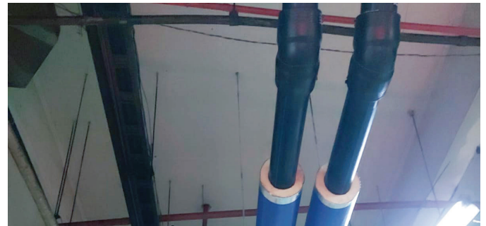
Post-insulated PE pipes for chilled water line at WalterMart Makati branch
