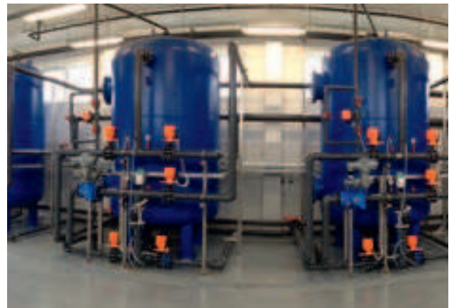
Sandfilter drinking water plant, Virovitica, Croatia
