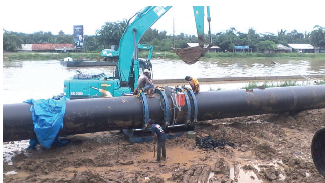
(1200mm pipe, siphon water project)
