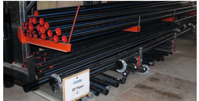
GF pipes on site, data center construction near Zurich (Switzerland).
