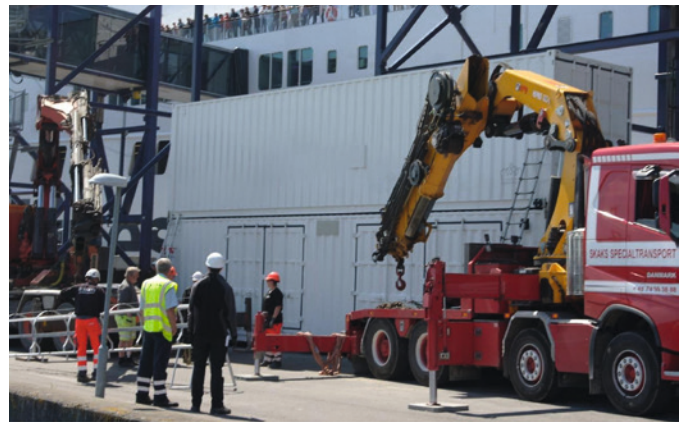
Containerized MarinePaq onshore installation at the port in Denmark.
