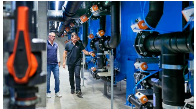
A wide range of manual, manual and actuated valve solutions from GF regulates the filter systems.
