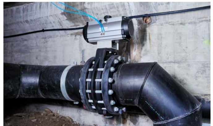
Successful underground test installation of the Butterfly Valve 565 Big in DN400 in the outdoor area of the Schlossbadi.
