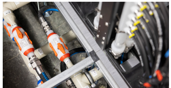
LiquidCore is engineered for efficient cooling in the white space, and its polymer components ensure ultimate coolant purity.
