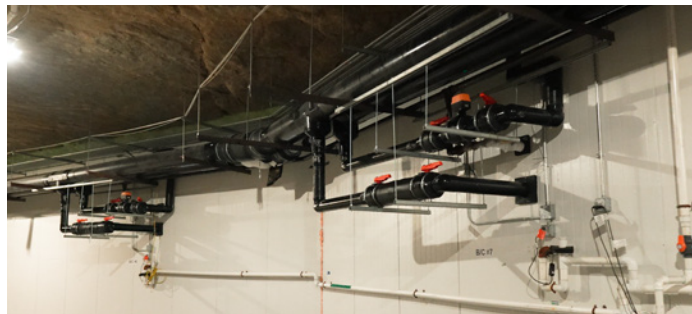
COOL-FIT 4.0 piping combined with GF valves delivers optimal cooling performance and efficiency for the underground cold storage facility.
