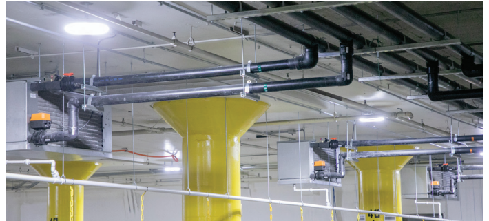
COOL-FIT® PE Plus piping combined with GF valves delivers optimal cooling performance and efficiency for the underground cold storage facility.
