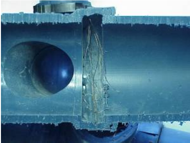
Pipe was not inserted to the pipe stop!
