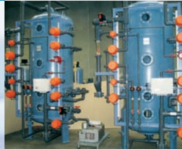
Demineralisation System in PVC.
