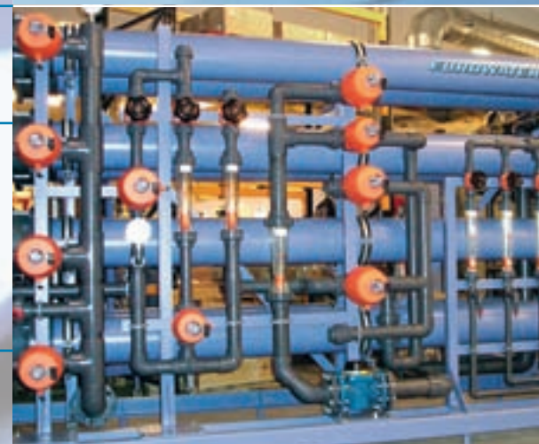
Reverse Osmosis in PVC-U.
