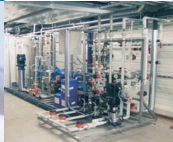
SYGEF® PVDF with BCF® fusion in Pharmaceutical Chemical dosing application.
