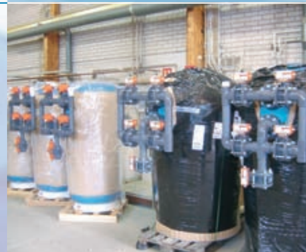
Water Treatment system for Ship Building with PVC-C and PE 100 piping and actuated valves for process control.
