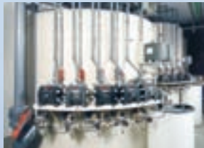
Chemical Injection System
