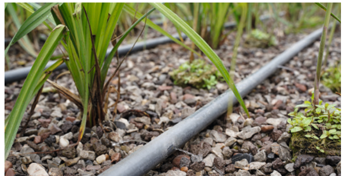
The charging facility comprises multiple pipes laid approx. 40 cm apart and uniformly perforated in order to distribute the wastewater on the surface of the wetland.
