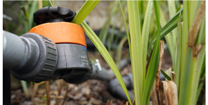
Those in charge are equipping the pilot installation with resilient and durable PVC-U pipes and fittings from GF Piping Systems.
