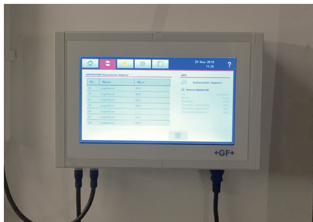
The integrated sanitary technology is easy to operate from the Hycleen Automation Master control unit. The panel is connected to controllers, which precisely control the individual valves and sensors.
