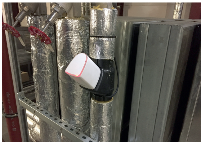
The retrofitted Hycleen Automation System guarantees reliable drinking water management at consistent temperatures above 55°C and a hydraulically balanced installation.
