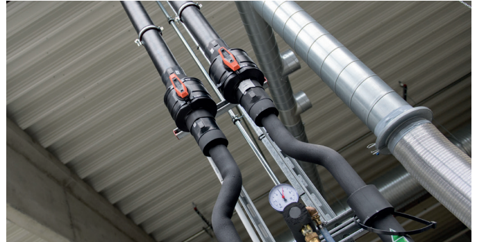
The ball valves type 546 in use in the printing house.
