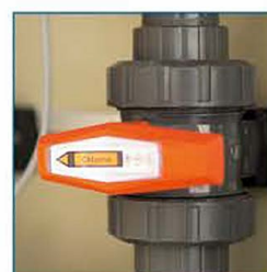
Ball valve labeling
