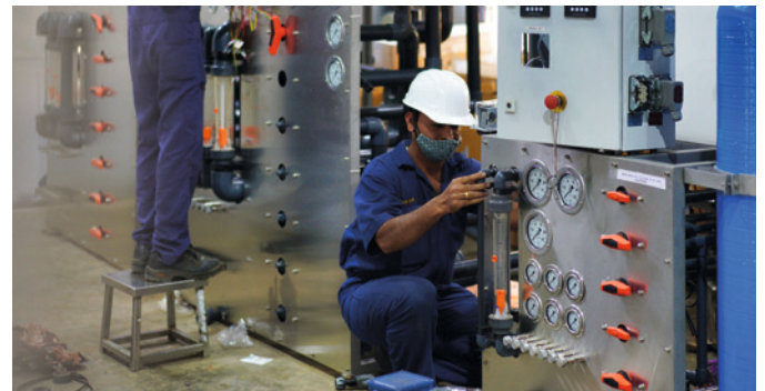
With the solutions of GF Piping Systems, Rochem's plants can treat up to 200.000 liters of water per day.
